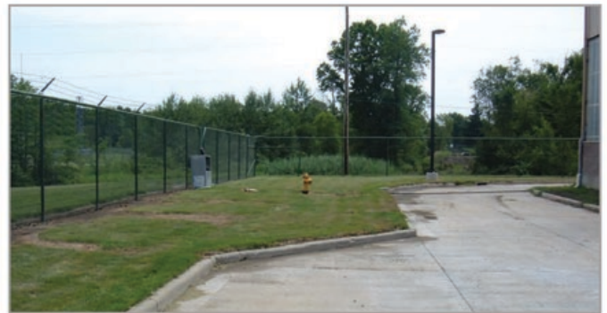
Stanchions Mounted on Perimeter Fence
